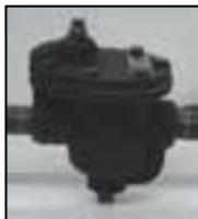
Uncovered Steam Trap
